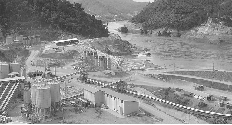
Xayaburi construction site 1,260 MW, wide angle view, year 2014: the first hydroelectric dam in the series of projected 12 dams on the mainstream of the Mekong in Laos, started in 2012, projected date of completion and operation 2018 [source: Tom Fawthrop]
