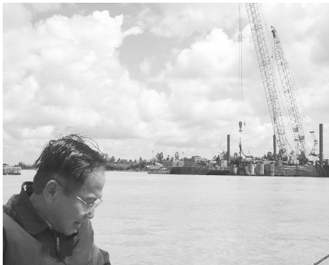
Crossing the Hậu River to visit construction site of the Cần Thơ Bridge
