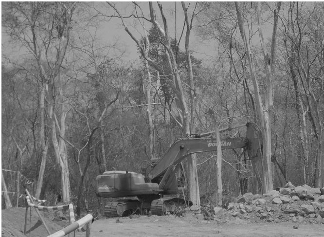
Don Sahong Project, deforestation of construction site with bulldozers for clearing ground [photo by Tường Năng Tiến]
